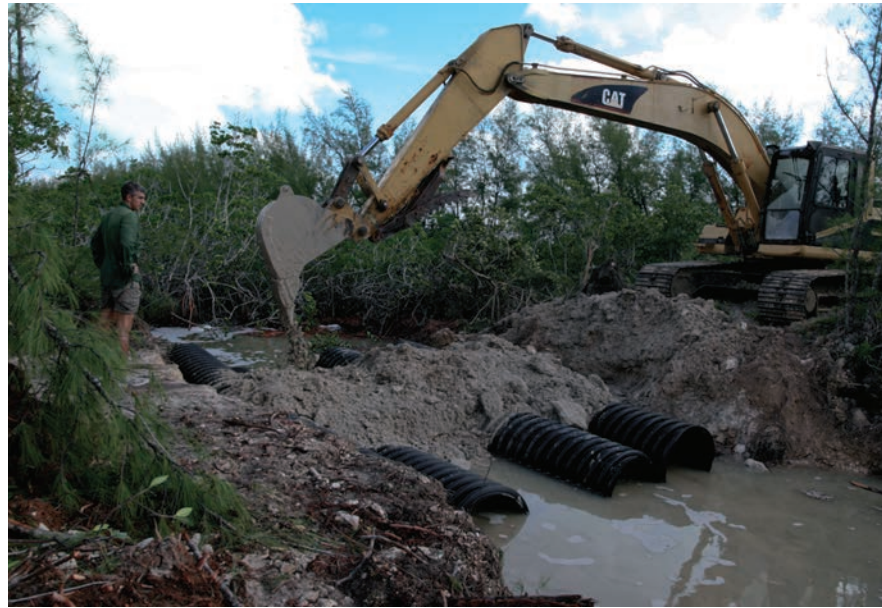
Fig. 8.21 Installing culverts under roads increases hydrologic connectivity between wetlands and the ocean. These projects are a common form of ecosystem restoration in The Bahamas. Photograph courtesy C. R. Layman.
