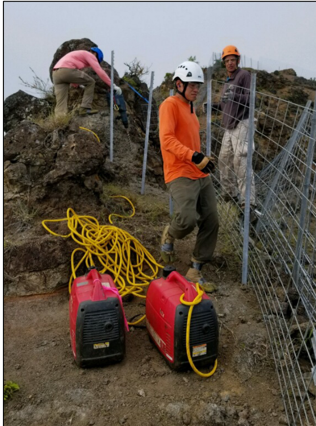
Using the Rock Hammer Drill to install a new section of fence
